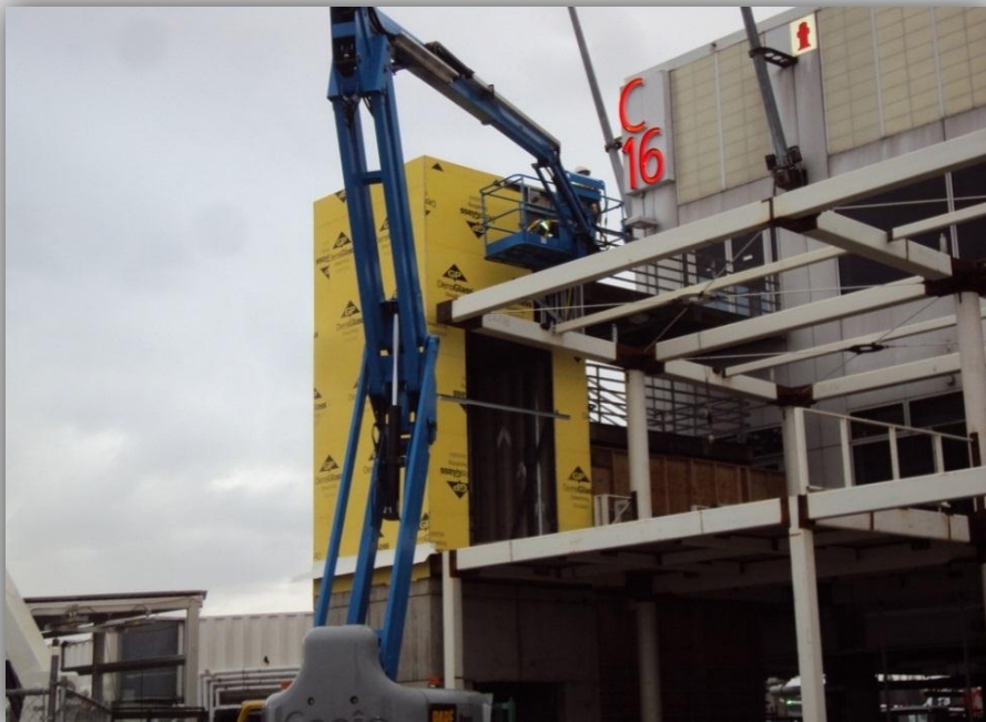
C16 Elevator Shaft & Panels
