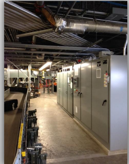
C88 Motor Control Panels operating
